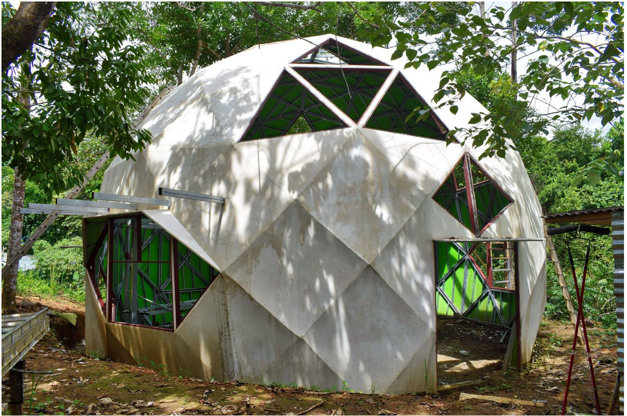
Geodesic Dome Frame House of 11 meter in diameter with metal reinforcement and panelling and plaster on the exterior. This home is still in construction. The geometry of the dome is a very interesting one which allows a spacious second floor.
